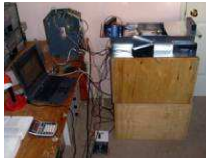
Control and Monitoring
